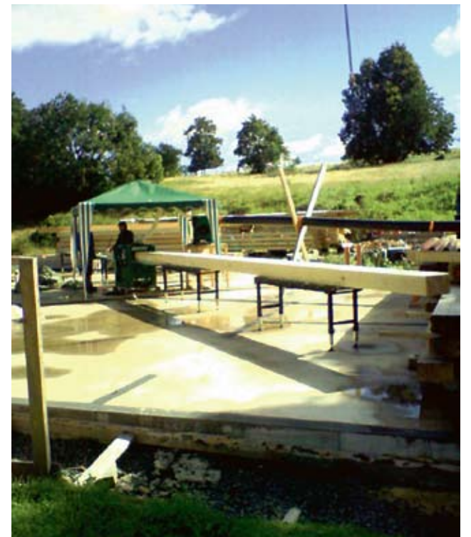
This is the photo that Per-Arne took with his cellphone, showing the planing of a 12 metre long beam with the measurements 8" x 12".
