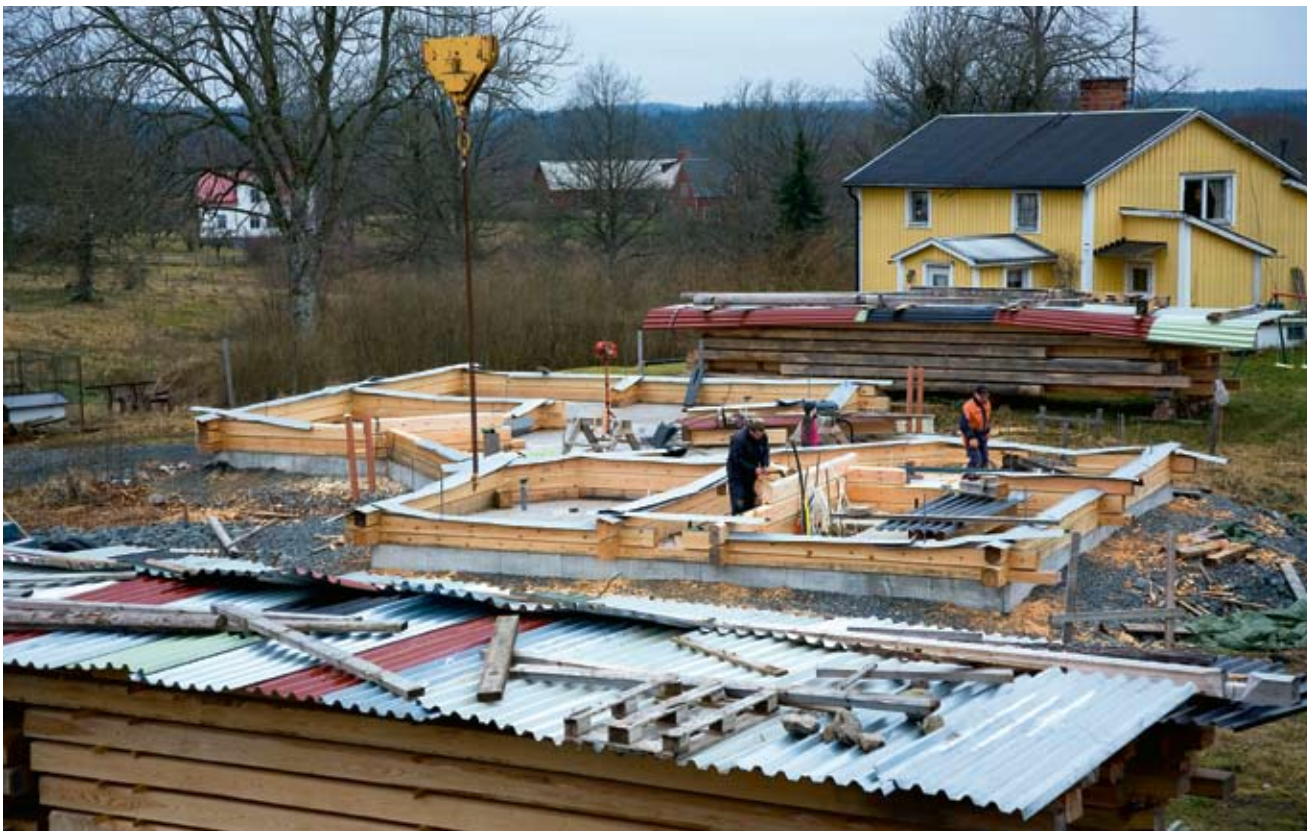
Per-Arne Ragnarsson and Peter Hall are building a log house of 270 square metres.
